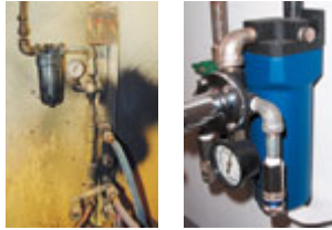
Figure 2. Various fittings and plumbing arrangements.
